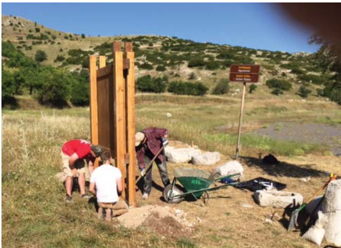
Top left: Students celebrate the successful installation of the Trail of Pan marker. (L-R: top: Kyle Mahoney, Vasilis Barkoulas, Asher Caplan, Matt Pihokker, Pat Playdon. bottom: Lauren Dreyfuss, Alex Weber.) Top right: The supply march to install posts in the middle of the Trail of Zeus. Middle: Kyle Mahoney and Matt Pihokker mix concrete for the post. Bottom: Matt Pihokker, Kyle Mahoney, Pat Playdon installing the Kiosk near the hippodrome.
