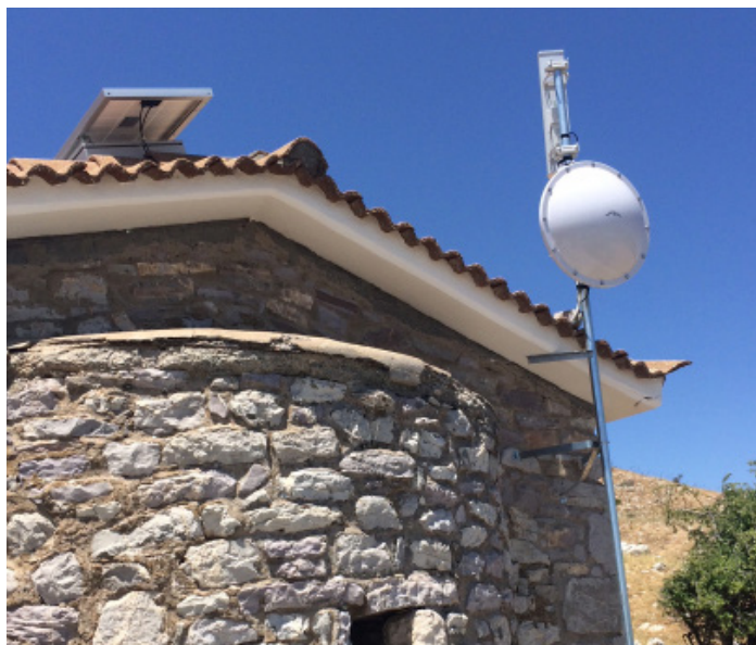
Below: The high-speed internet antenna and solar panels at the church of Profitis Elias.
