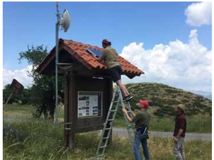
Kyle Mahoney, Tom Keating, and Ryan Culpeper Setting up the Hippodrome internet installation.
