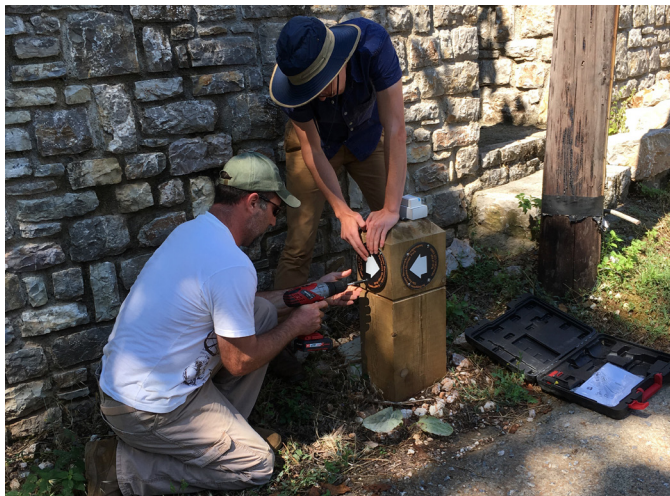
Above: John Keck and Buck Roberson installing directional signs on the Trail of Pan
