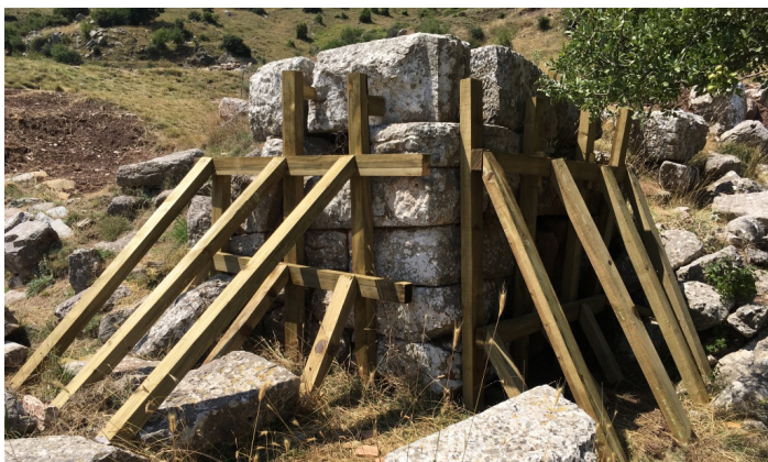
The wooden lattice construction at the northeast corner of the Administration building
